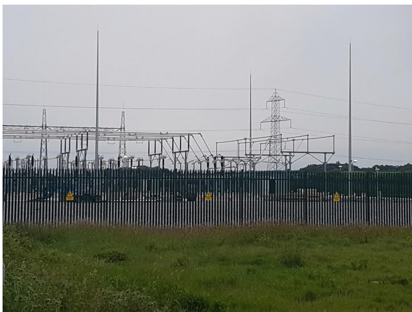
Figure A2-6.1 Typical Example of 220 kV Substation
